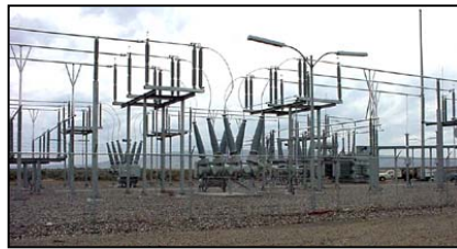
Fig. 2. Electrical Substation and Transmission Lines
