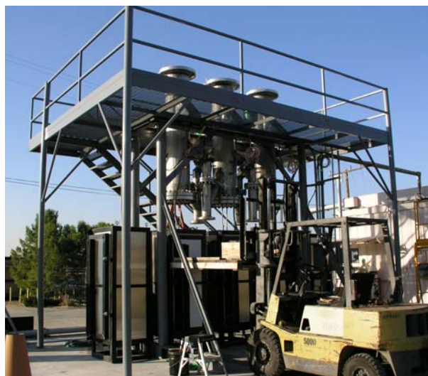
Figure 5. Reactors assembled on support framework.
