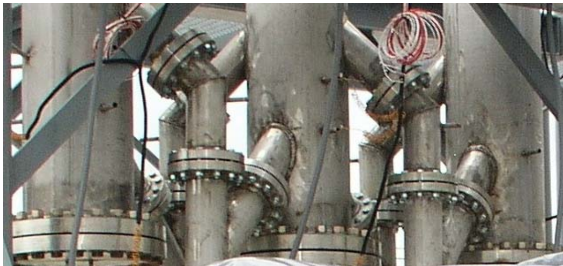
Figure 6. Assembly of solids transfer legs connecting the three main reactors.
