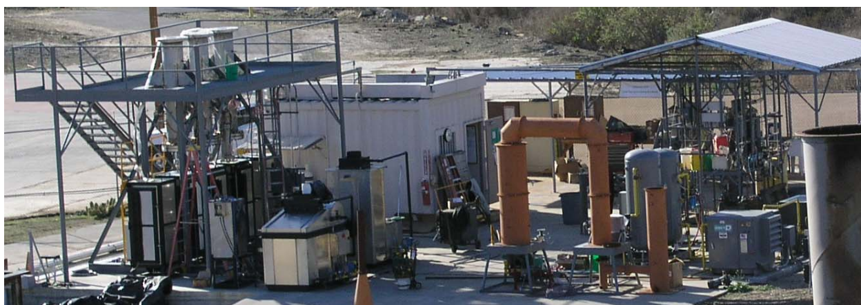
Figure 11. Photo of assembled pilot plant system.
