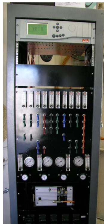
Figure 9. CEMS rack with controls for product and calibration gas flow to analyzers.
