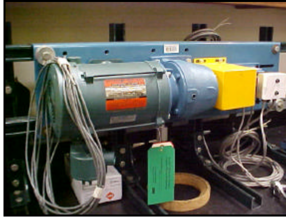
Figure 6. Explosion proof motors and pumps are used throughout the Hydrogenation Facility.
