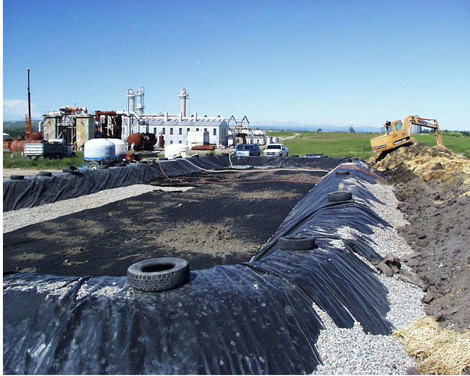
Photo 5. Contaminated soil being mixed with straw, storage tanks for additives and leachate collection on the southwest side of biopile cell.
