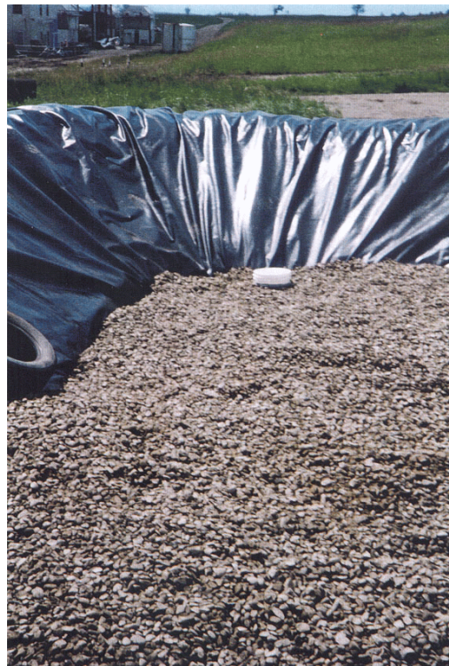
Photo 4. Leachate collection pump in the Southwest corner of the biopile cell.
