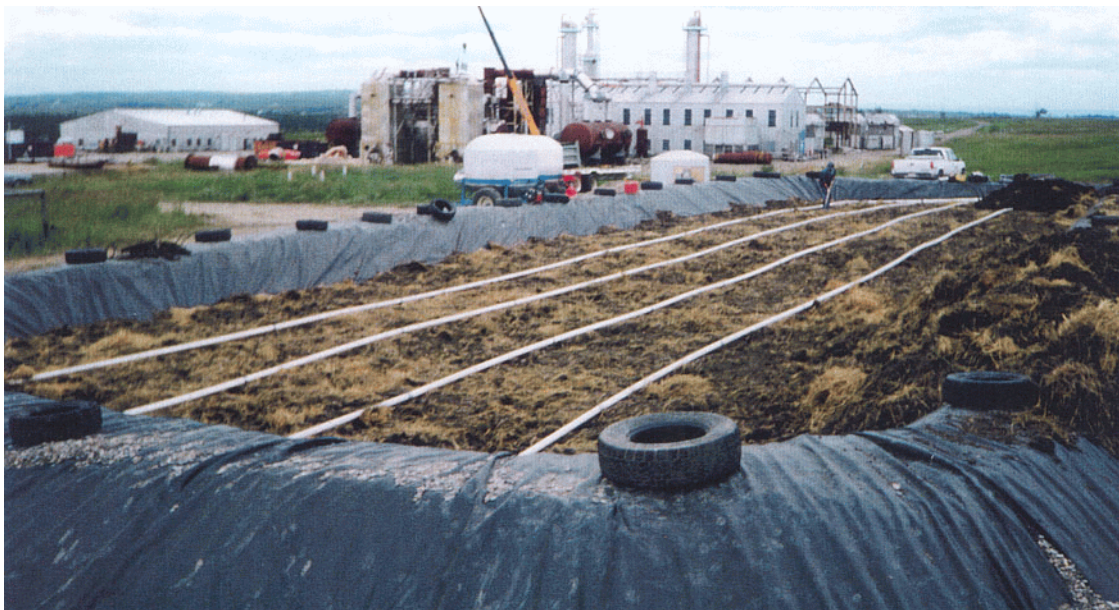
Photo 6. Aeration piping above the first 250 m 3 of contaminated soil and straw.
