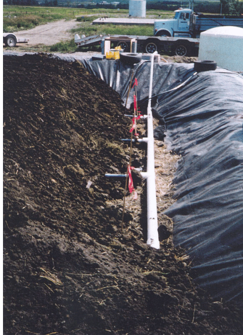
Photo 7. Aeration system header.
