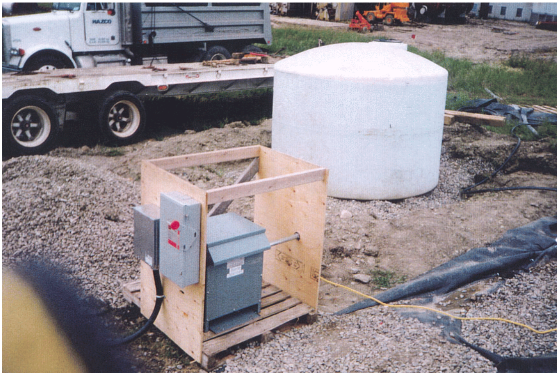
Photo 8. Close view of electrical supply and leachate collection tank on the southwest side of the biopile cell.
