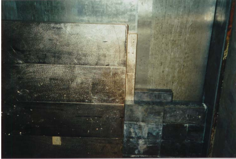
Figure 11. Detail of the bismuth gamma shield blocks, 5cm (2 in) offsets at the top/bottom and sides.
