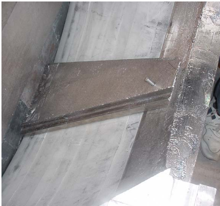
Figure 19. First stave in position. Note the partially inserted aluminum rod used to pin the stave to the collar. The bottom seven staves were pinned to the collar.
