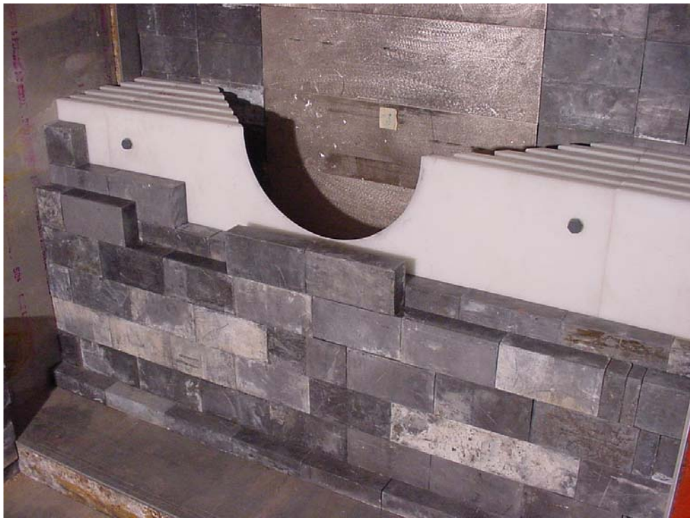
Figure 17. Lower half of the polyethylene in position, lead bricks to the bottom half-collar.
