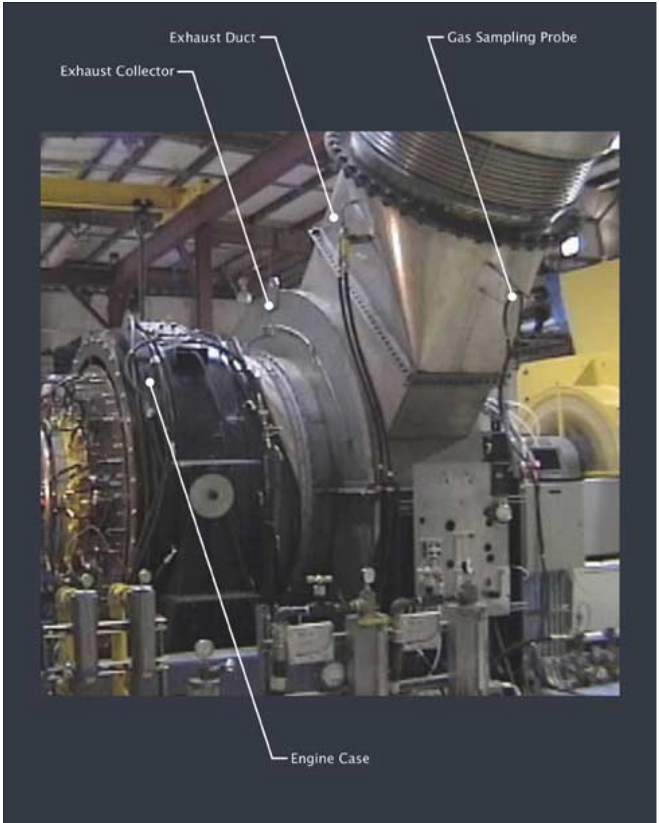
Exhaust Duct and Engine Case
