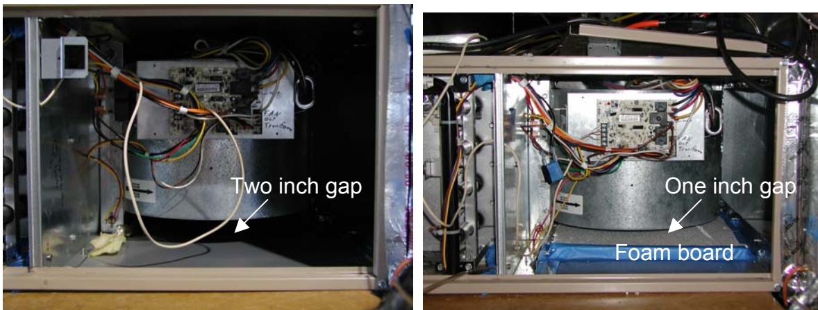
Figure 6. Standard fan in cabinet with no restriction (left) and with added foam board restriction (right).
