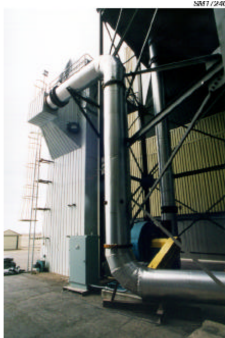
Figure 1. AHPC unit installed at Big Stone with new inlet ducting and side transition inlet configuration.
