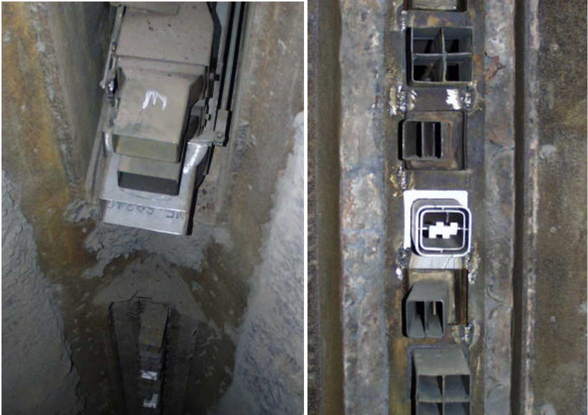
Figure 6.3-4: Photo of Installed Firing System Components.
