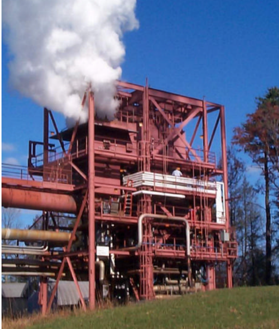
Figure 6.3-6: The BSF in Operation During Testing of the MVB Coal.
