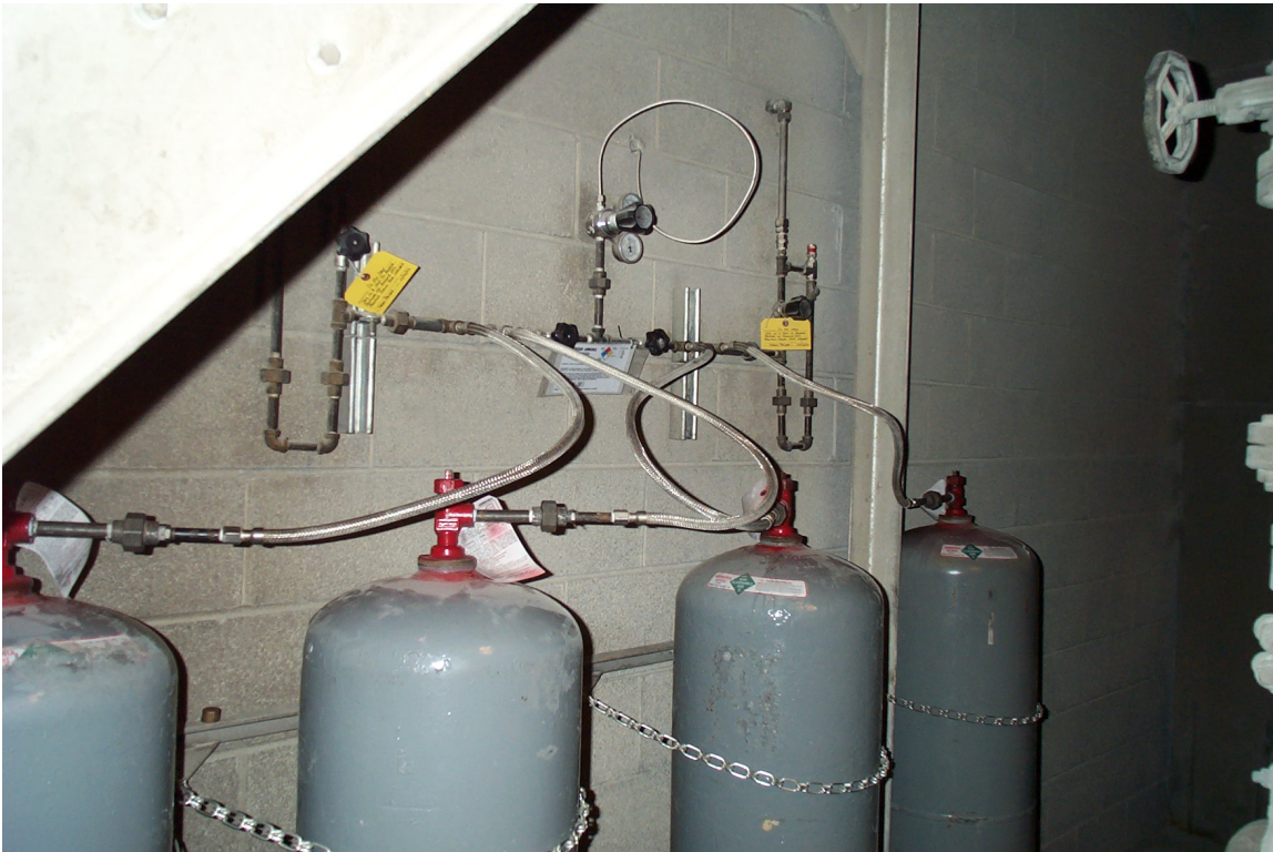
Figure 13. Four 150-lb ammonia cylinders connected to the ammonia supply manifold in the Unit 1 Fan room.
