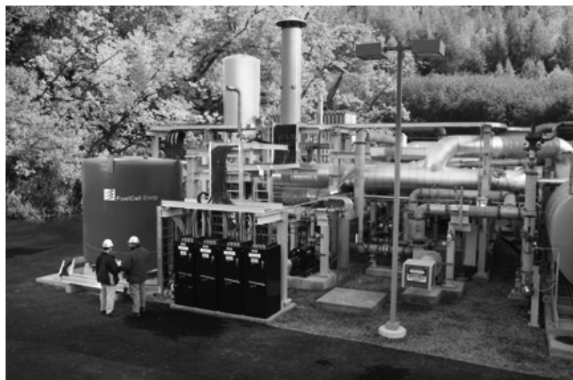
Figure 11. MEGAWATT TESTING AND CONDITONING FACILITY: Fully Ready for Conditioning and Testing
