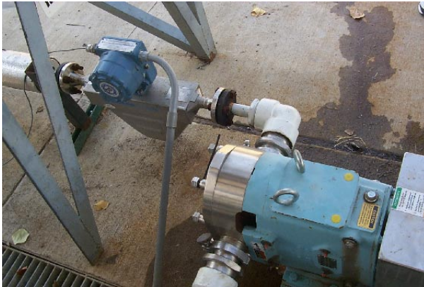
(b) Variable frequency pump (0~2000GPM)
