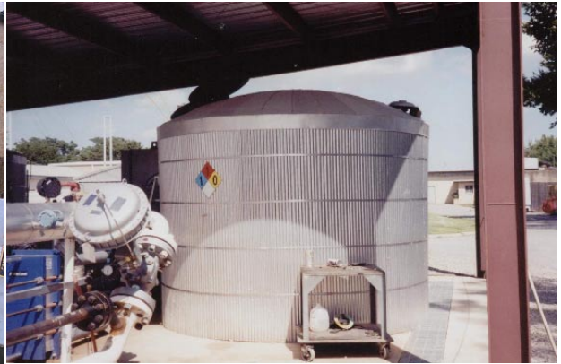
(c) Water tank for outdoor flow testing loop
