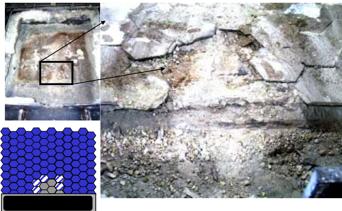
Figure 15 – Pilot Cell 2 Post Operation Tile Condition
