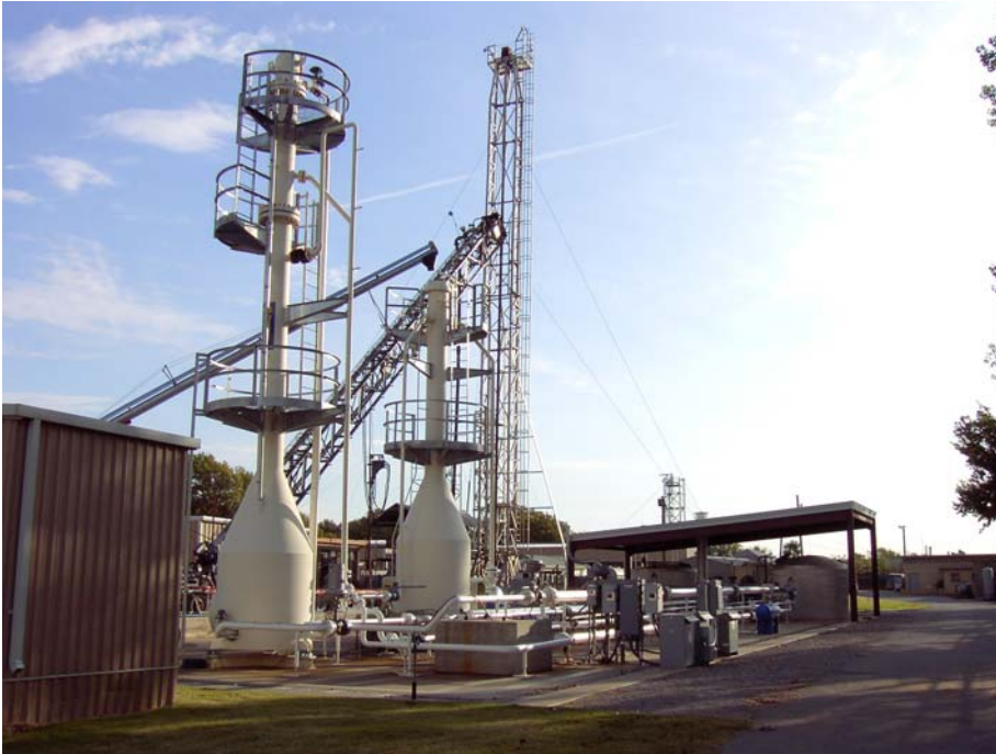
Figure 3.1 - Cuttings Injection Hopper (right) and Separation Tower
