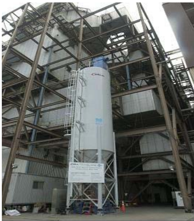
Fig 1. Carbon Injection Storage Silo and Feeder Trains Installed at PPPP.
