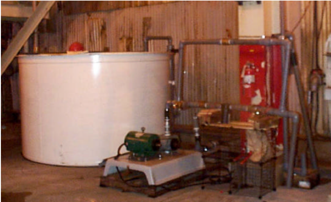
Figure 5 Pilot Plant at Simpson pulp and paper mill
