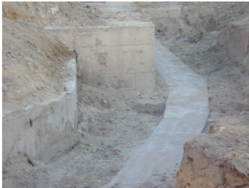
Figure 7. The underground electrical duct running along side the south cooling duct
