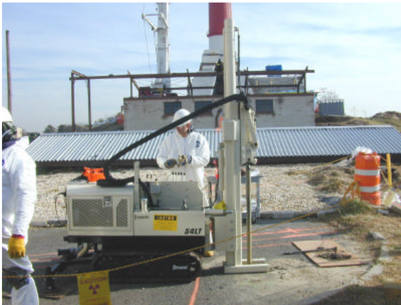
Figure 5. Geoprobe® Model 54 LT continuous push soil-probing unit used to install monitoring ports in soil adjacent to the BGRR Below Grade Ducts
