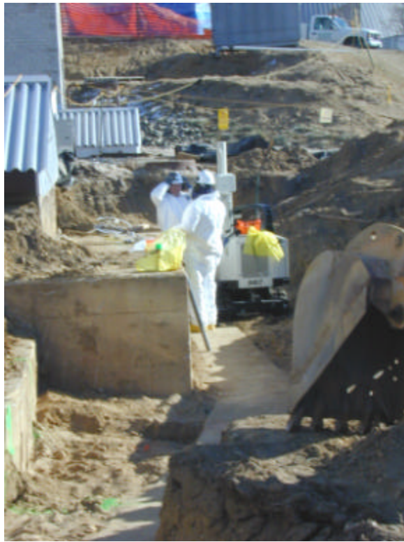
Figure 8. Geoprobe® installing ports along the south duct, between the electrical duct and main duct
