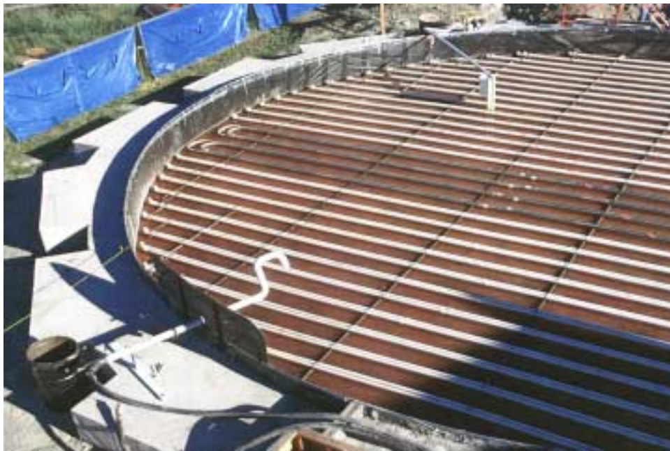
Figure 3.11 Tank basin showing location of cooling coils
