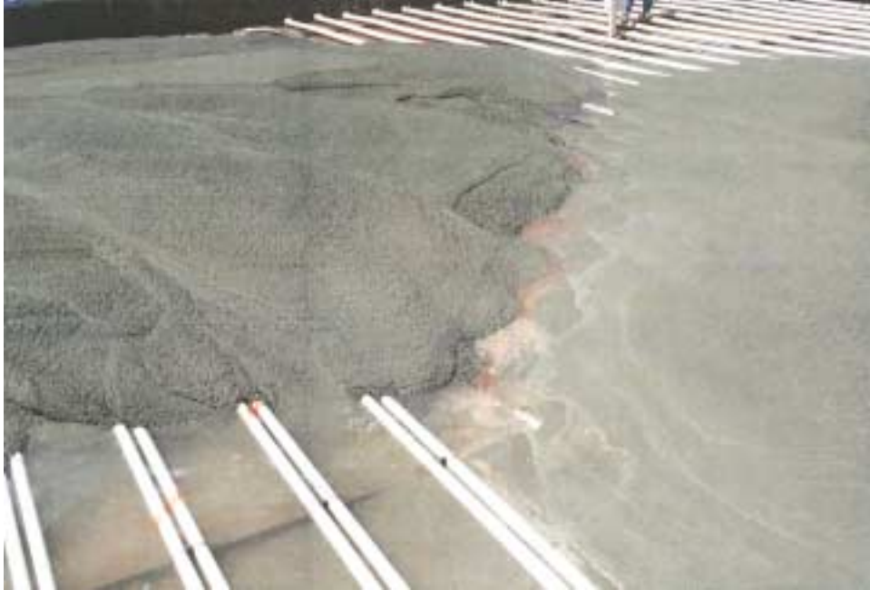
Figure 3.12 Pouring grout over the tank bottom to direct fluid to the steam jet entrance
