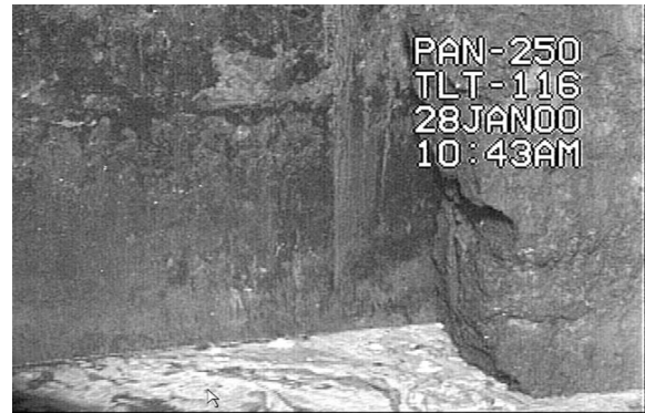
Figure 4.2 Tank Wall Waste Retention After Transfer 2
