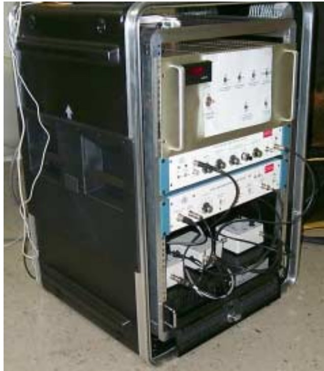
Figure 6.3. Tank Top Electronics
