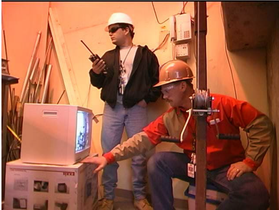
Figure 15 Operating GIF crane from behind temporary shield wall. (HP staff communicates with Control by radio. Crank used to swing crane jib. TV monitor shows position of liner.)
