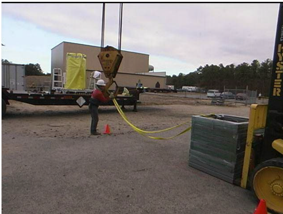
Figure 18 Rigger attaches rigging straps to Grove crane hook before exiting the high radiation area.
