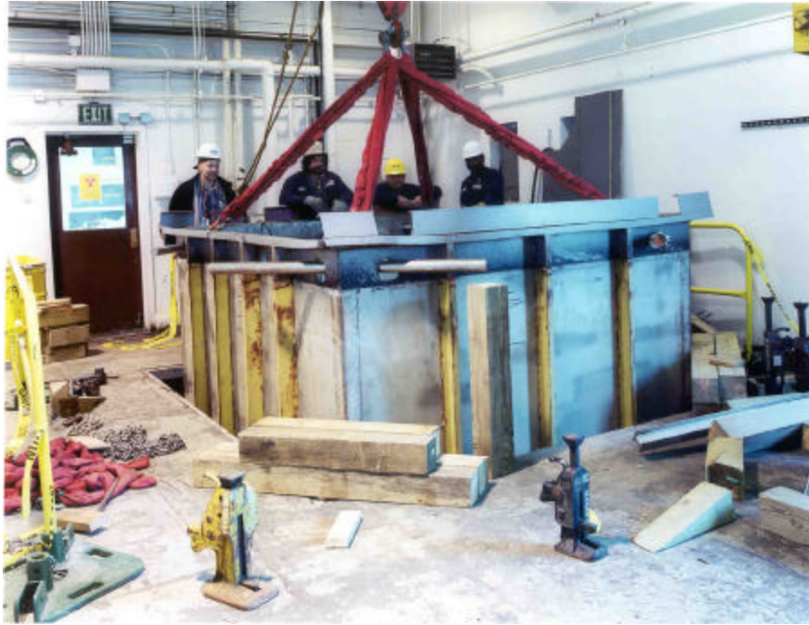
Figure 22 The jib crane was able to lift the tank after the backfill sand loosened up.
