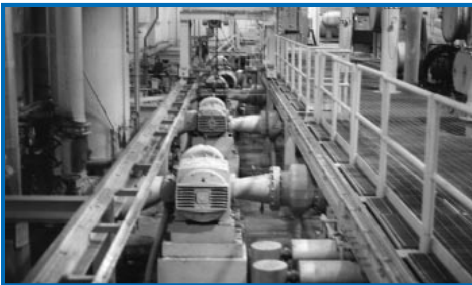
Motor system upgrades reduce energy usage at RCID's chiller plant.
