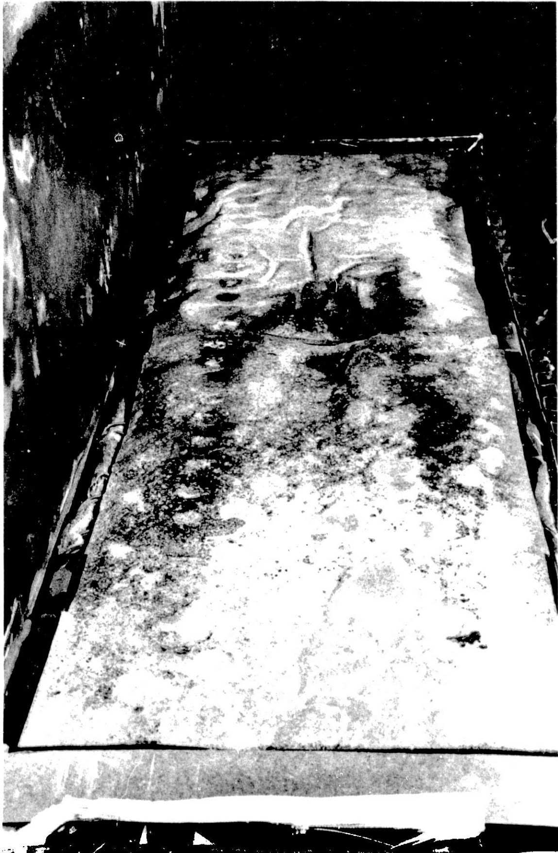
Fig. IV-27. View of Top Insulator Sheets
