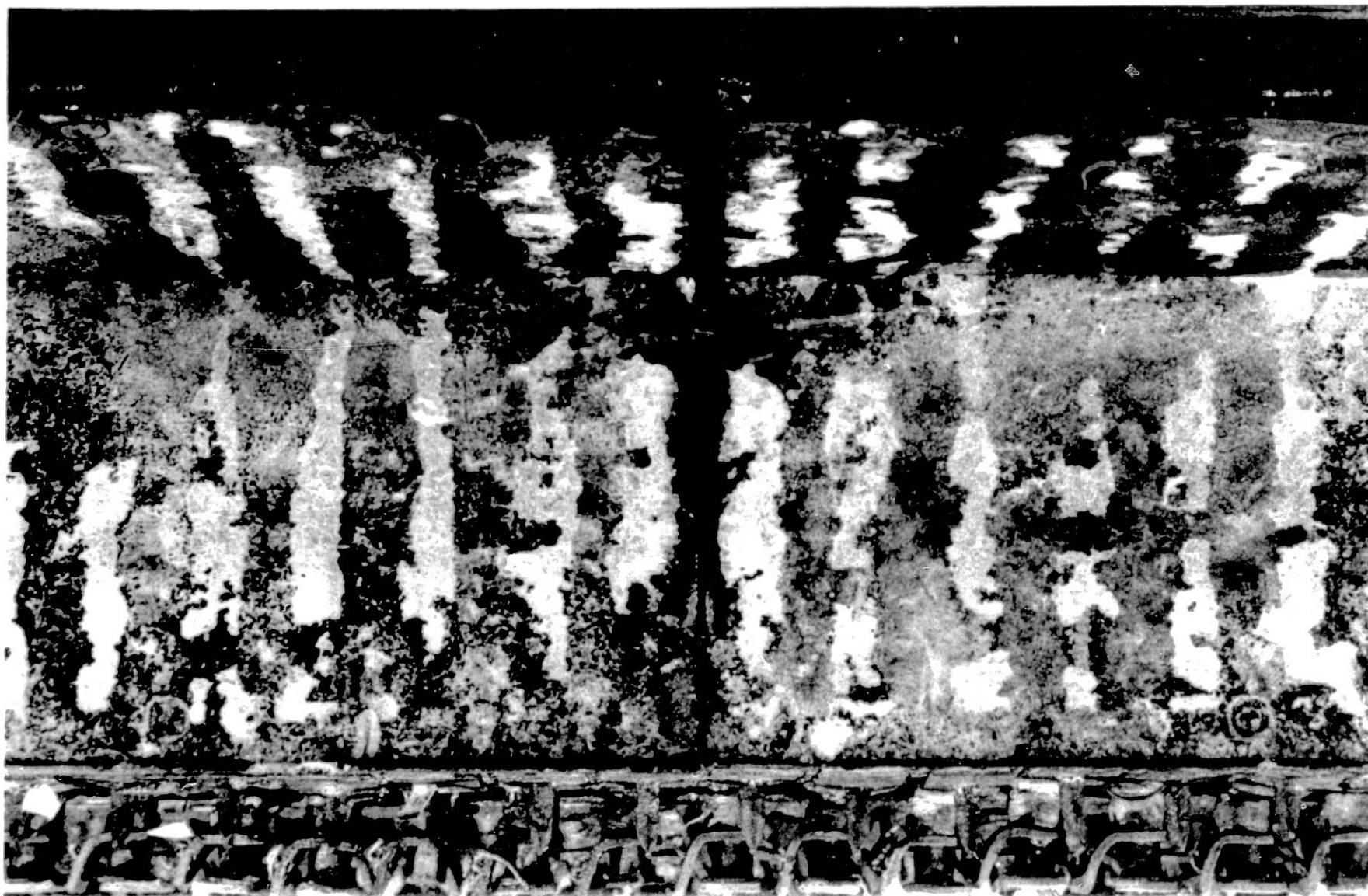
Fig. 17-30. Area of deteriorated insulation in Pool on st. 6111 and 16.
