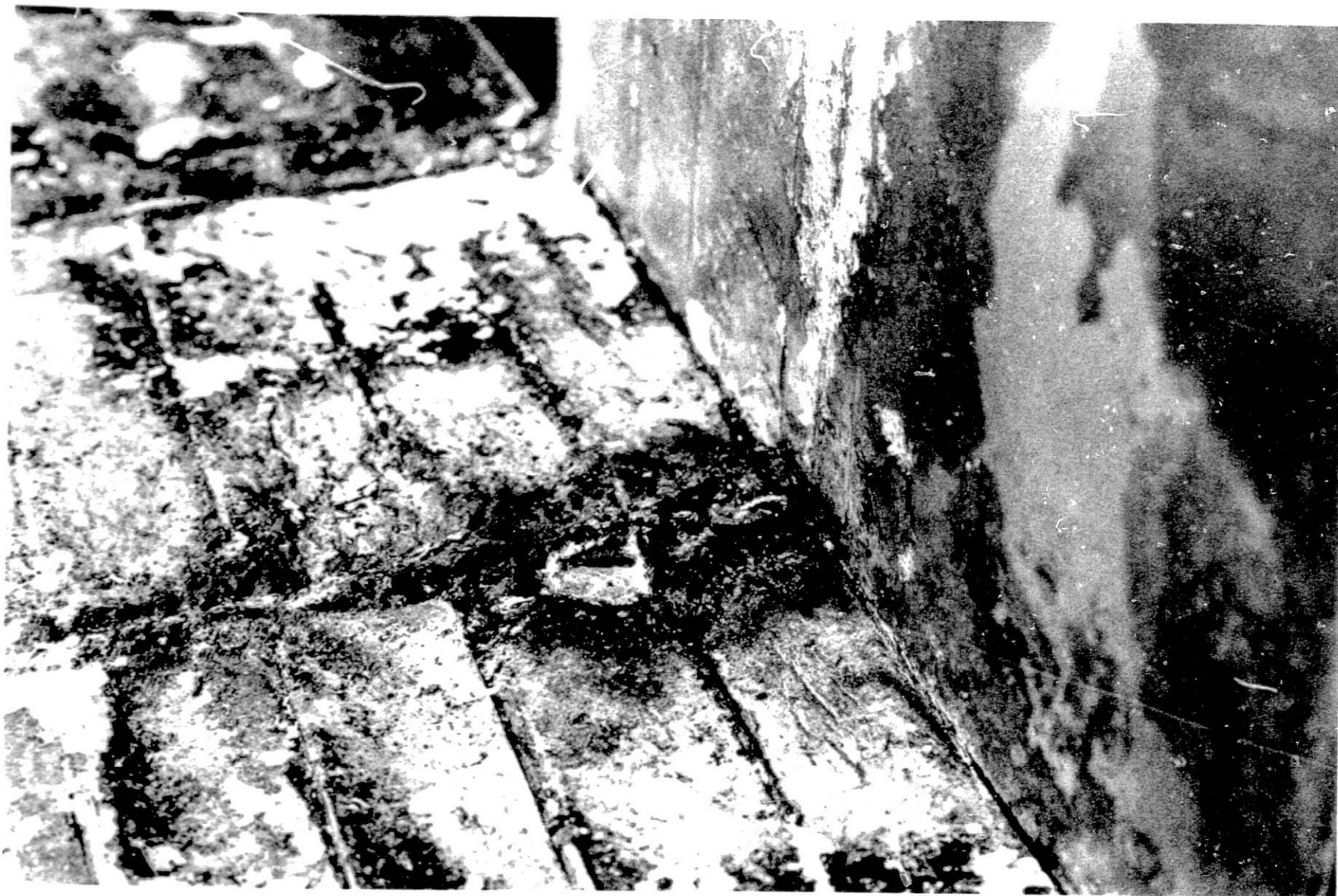
Fig. V-10. Lithium-Aluminum Alloy from Cell 2 (The Li-Al leakage occurred after the cell temperature had exceeded 600^{\circ}\text{C} and after the corrosion caused by the presence of electrolyte.)
