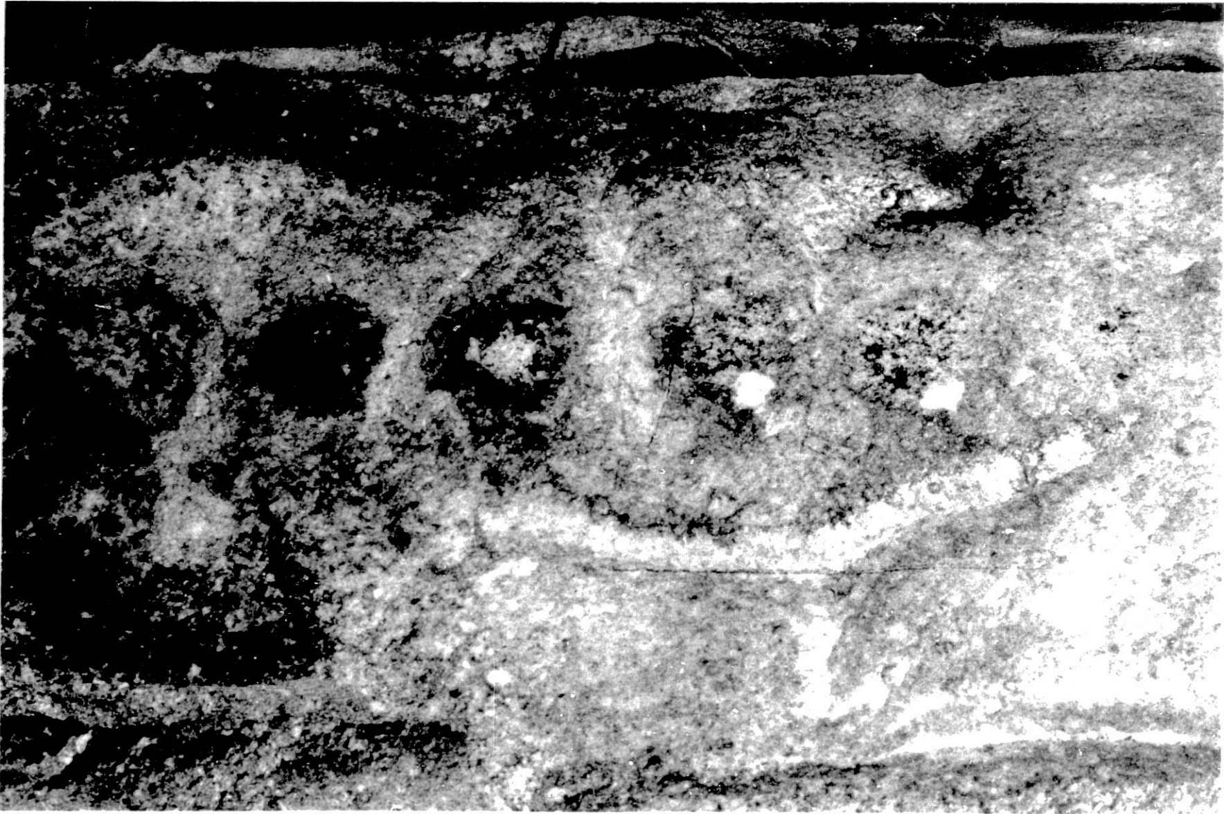
Fig. IV-28. Closeup View of Insulator Sheet Showing Crack
