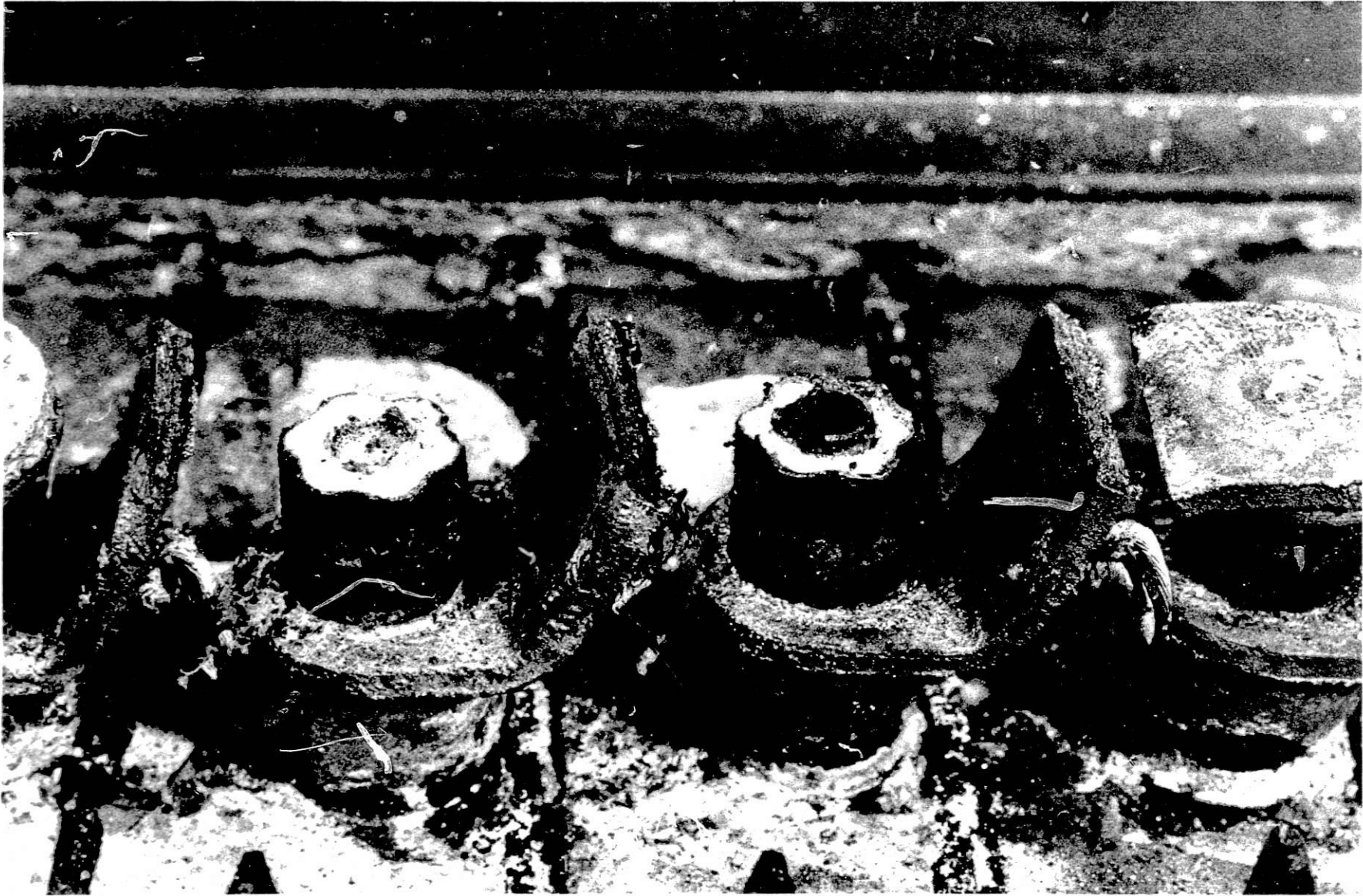
Fig. IV-34. Molten Positive Terminals and Molten Bridges across Insulation between Cells
