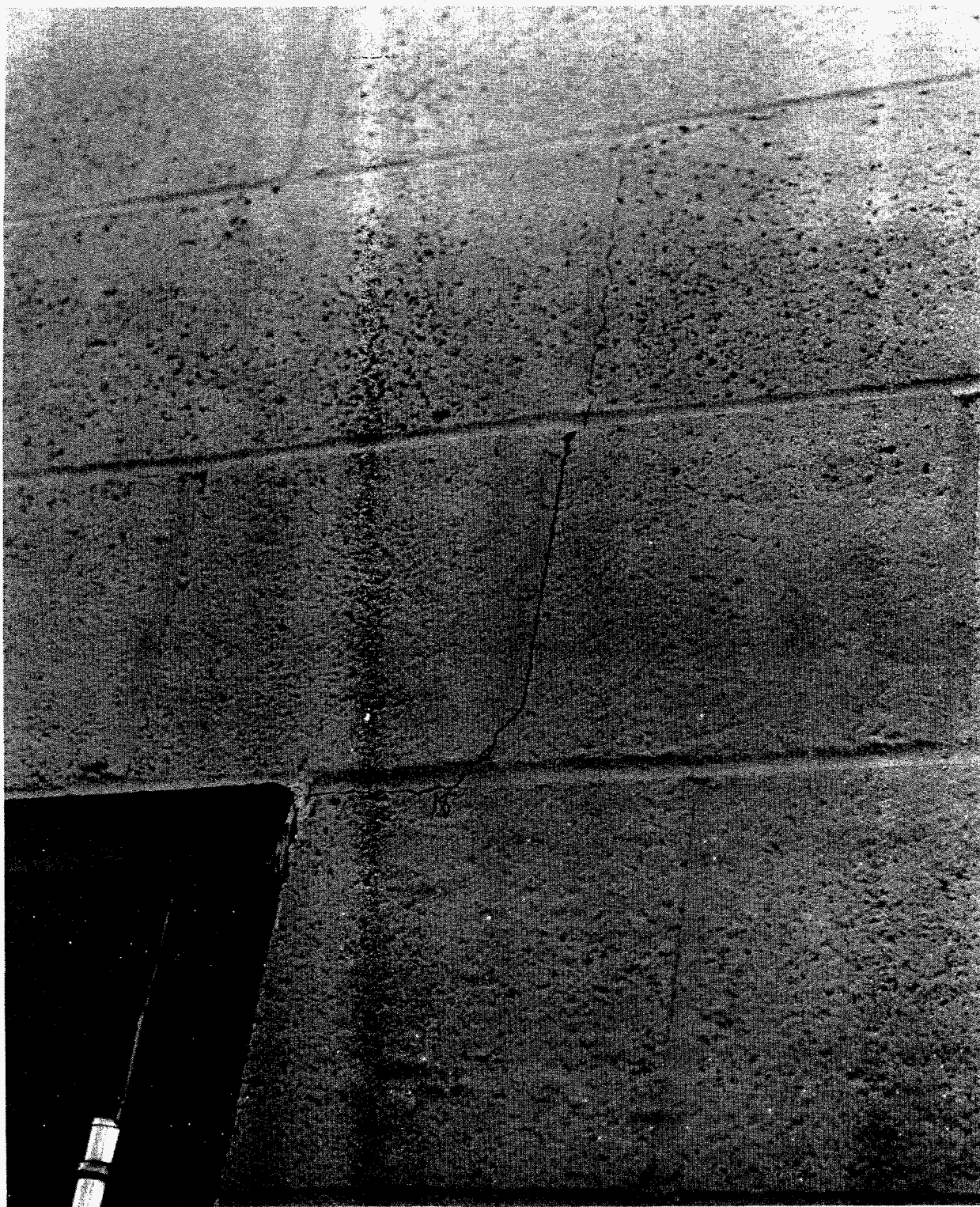
Fig. B-16. Building 701, north end of east side, crack over fan room door, 0.13 cm/sec.
