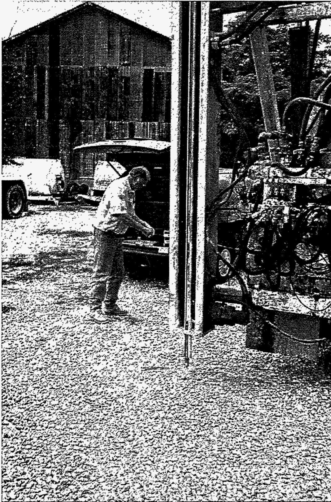
Figure 3. Lance injection truck with instrumented injection tip installed. Masthead is locked in the vertical position.
