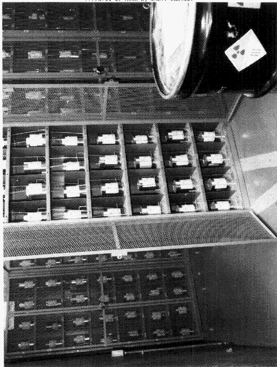
PPF/2736-Z, Room 2, Shelf Cubical
