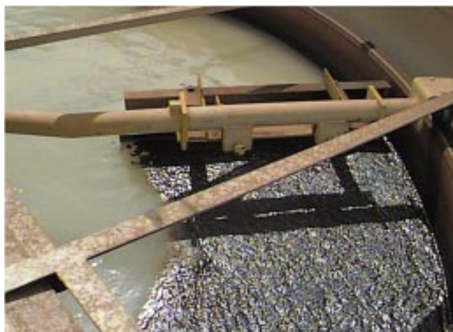
Figure 3. Contaminant floating on water in the dissolved-air-flotation tank (at lower right of Figure 2). Dissolved air forms bubbles that capture and lift free-product contaminant to the surface of the separator.
