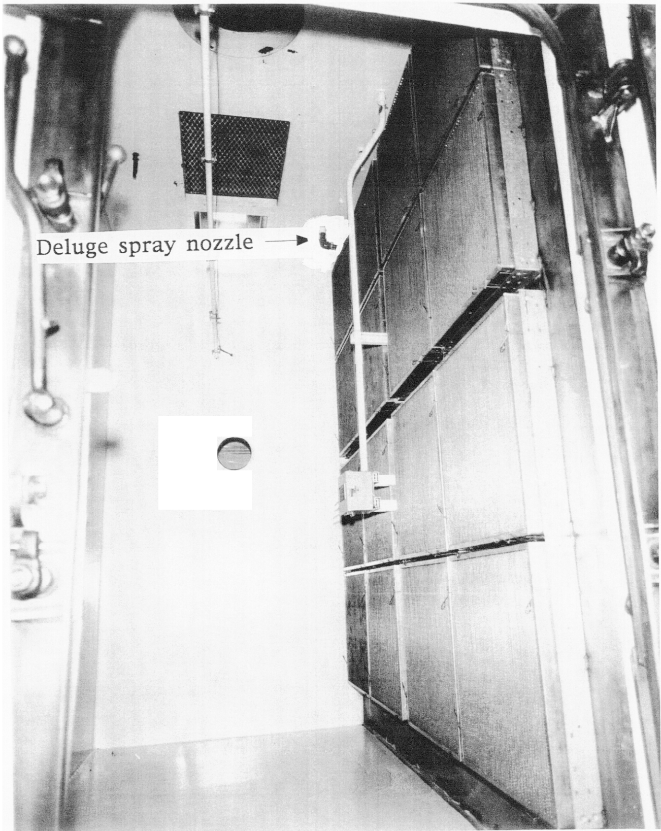
Figure 3. Photograph of a deluge spray nozzle mounted on the ceiling of a 4x4 HEPA filter plenum and located close to the inlet of the metal mesh demisters. The access door to the demister stage was opened for the photograph.
