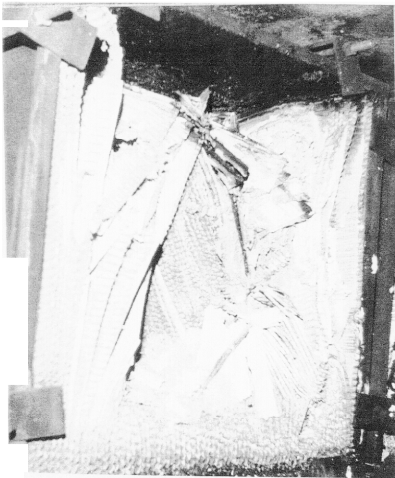
Figure 12. Photograph of the front side of a 3rd stage HEPA filter.
