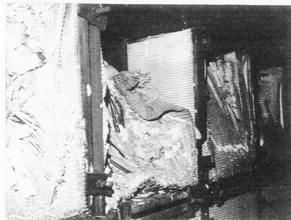
Figure 11. Photograph inside the middle chamber of the filter plenum showing the front side of the 3rd stage HEPA filters.
