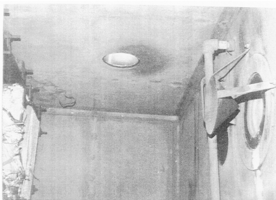
Figure 8. Photograph inside the front chamber of the filter plenum showing the air inlet with deflector cone and the damaged first stage HEPA filters.
