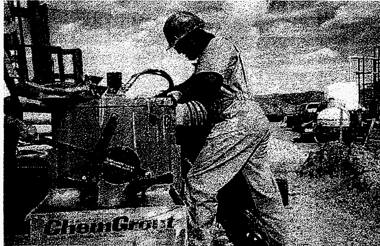
Figure 15. Mixing grout at Sandia. Photo shows grout being transferred from mixing tank to holding hopper.
