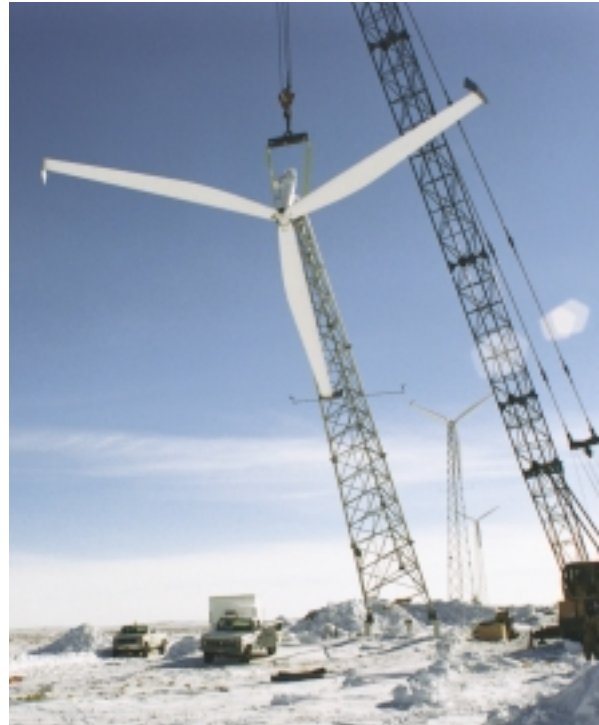
Seven new AOC 15/50 wind turbines are joining three wind turbines installed in 1997 near Kotzebue, Alaska. Kotzebue Electric Association and other Alaskan utilities are learning about how the wind turbines perform in the cold, harsh Alaskan climate.
