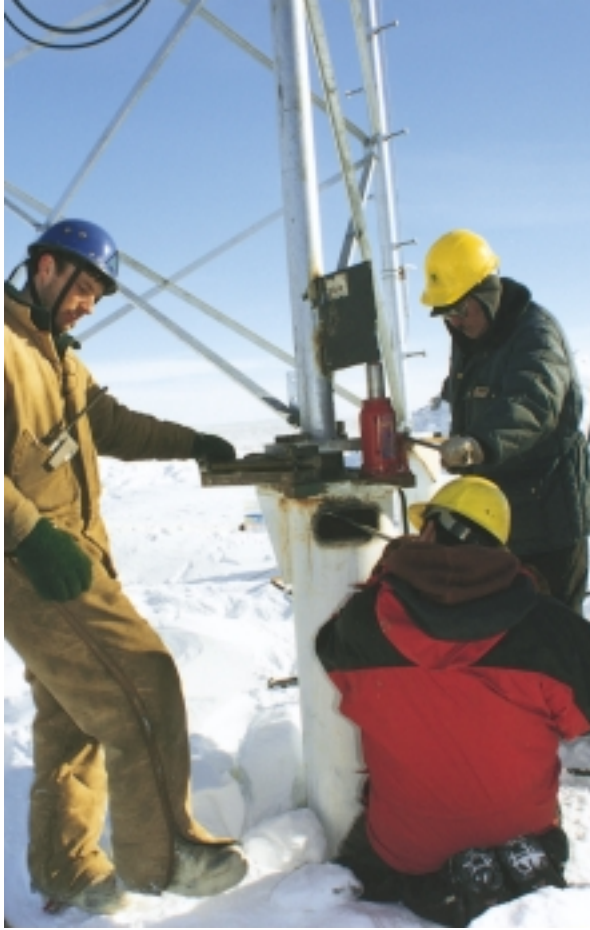
Workers attach one of seven new AOC 15/50 wind turbines to its foundation, specially designed to protect the tundra and underlying permafrost.
