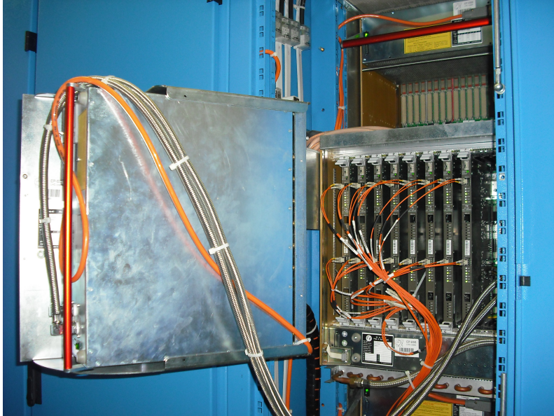
Figure 5.8: Picture of the rear part of a ROD 9U VME crate with the water cooled power supply and the TM.
