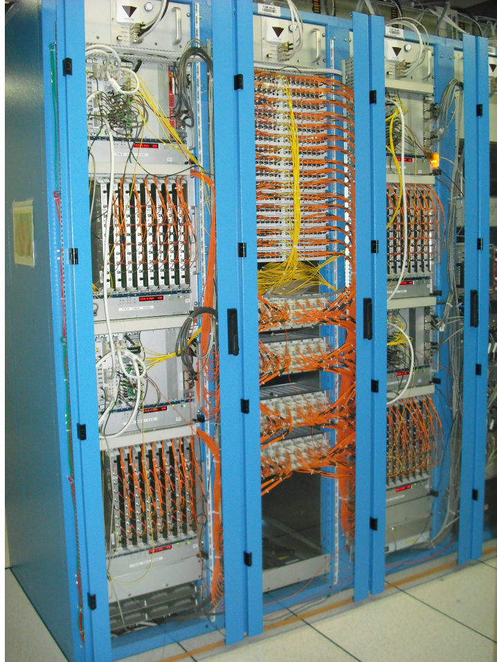
Figure 2.8: Picture of the TileCal back-end electronic crates at USA15.
