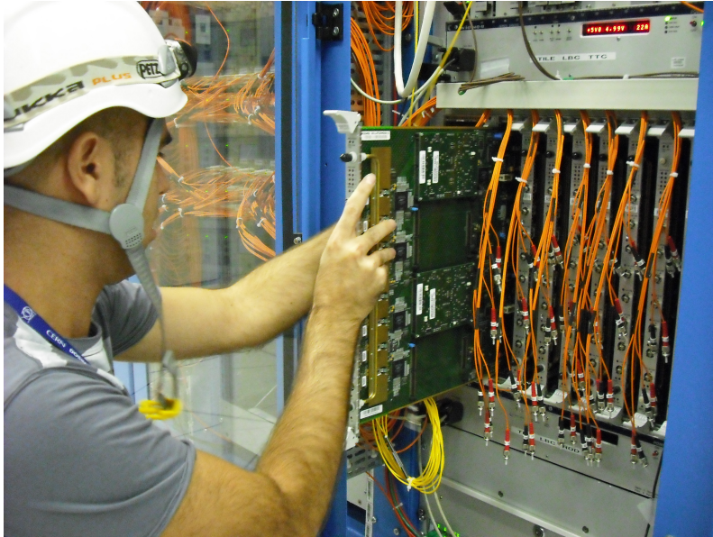
Figure 5.6: Installation of the ROD modules in USA15.
