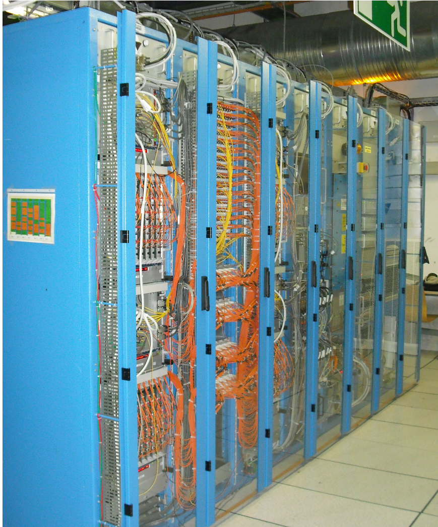
Figure 5.9: Picture of the TileCal back-end system racks in USA15.
