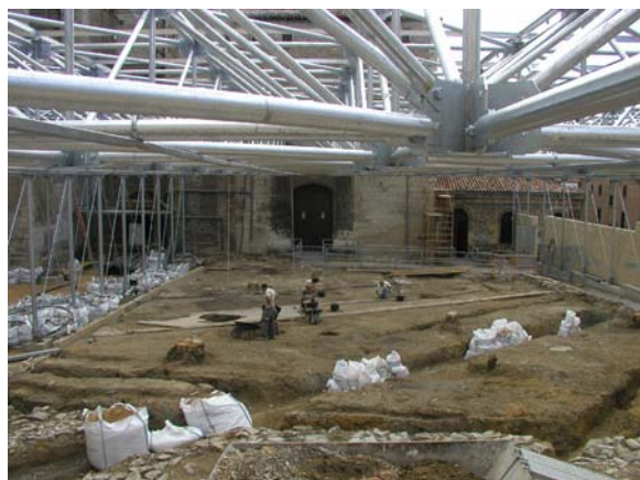
Figure 1. General view of the excavated medieval contexts in the exterior of the present cathedral of Santa María (Vitoria-Gasteiz, Basque Country).
