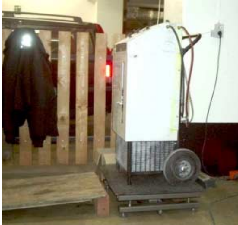
Figure 14: A recovery station Waeco RHS 650 on the scale before and after the recovery operation.
