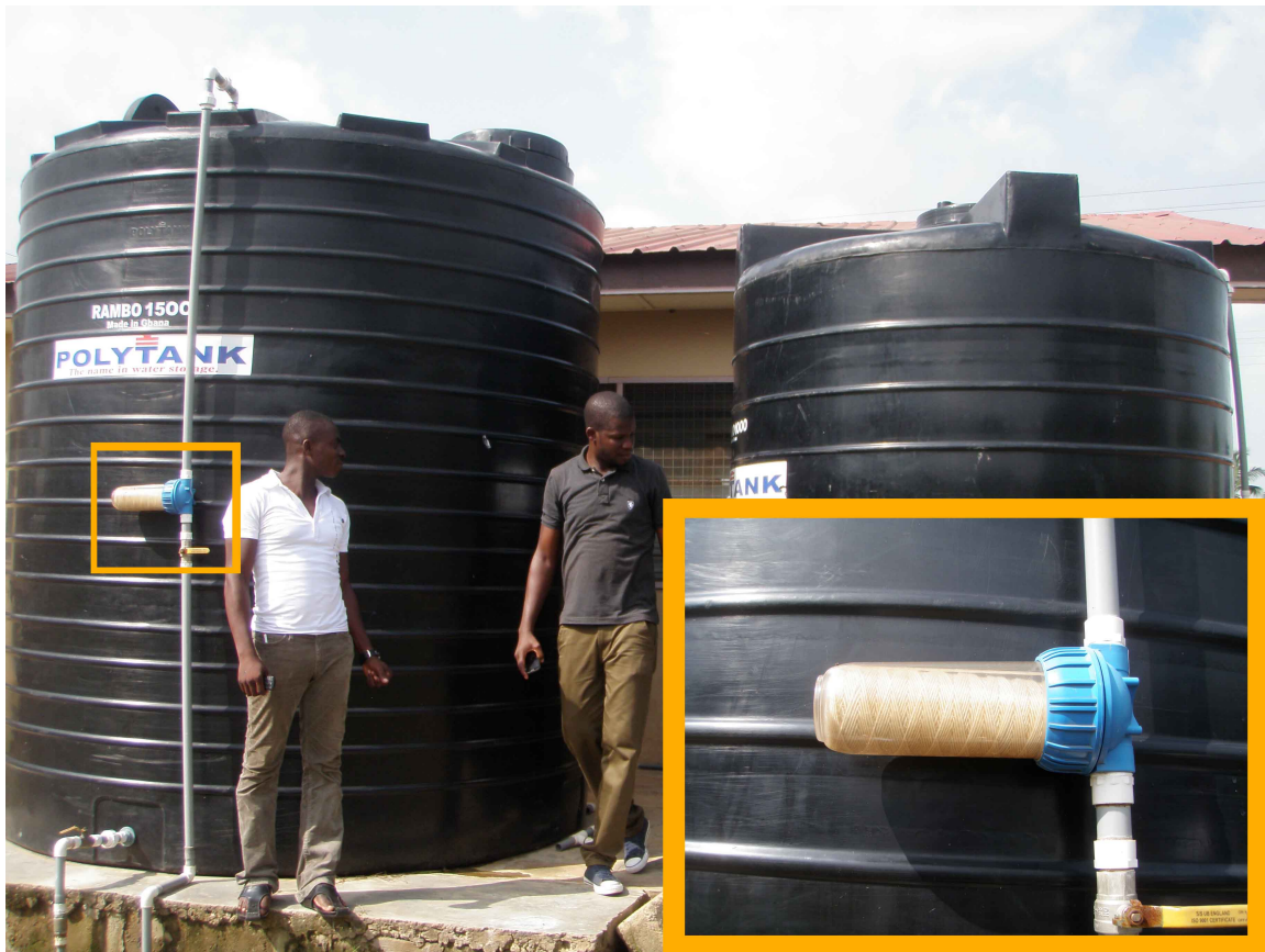
Holding tanks and external primary yarn filter situated outside a sachet water factory in Sogakope.
