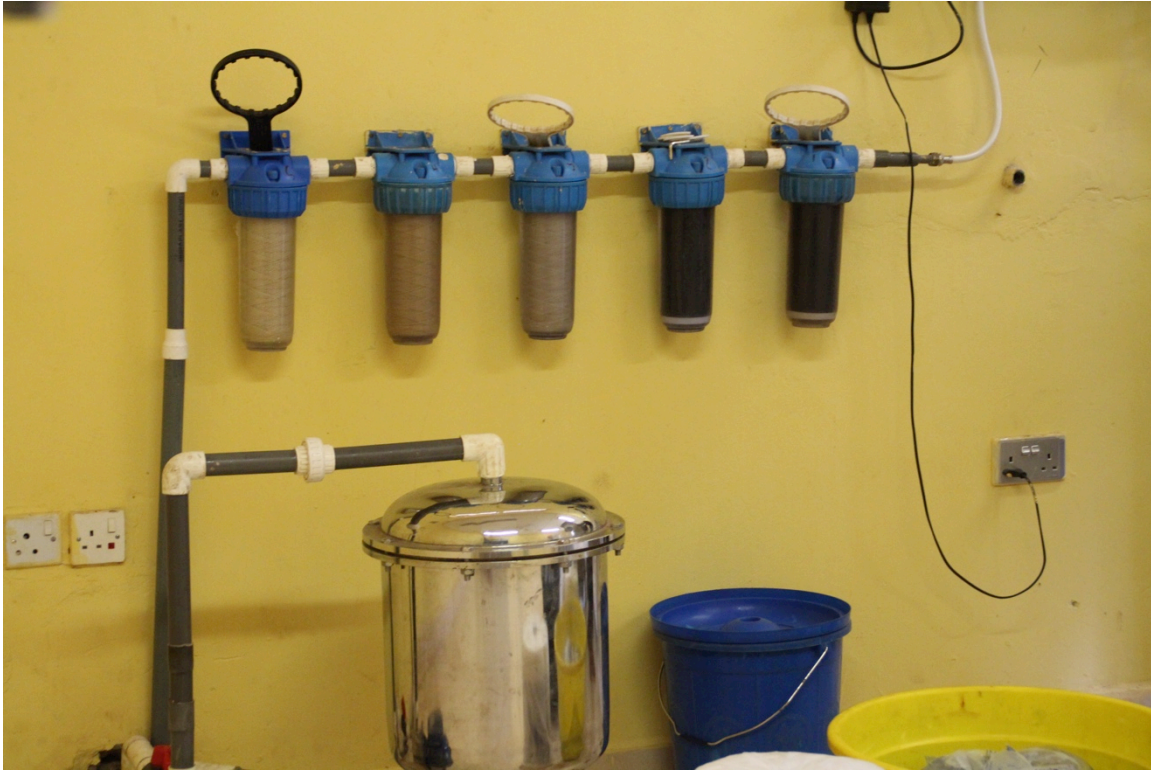
Below the set of yarn and carbon filters, this sachet plant employed the use of a clay filter
