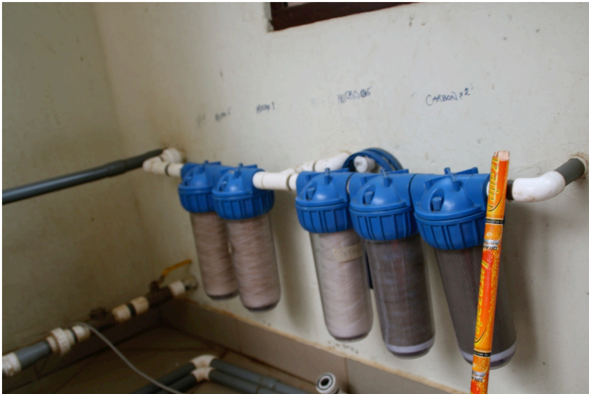
Three yarn and two carbon filters leading to sachet filling machines.
