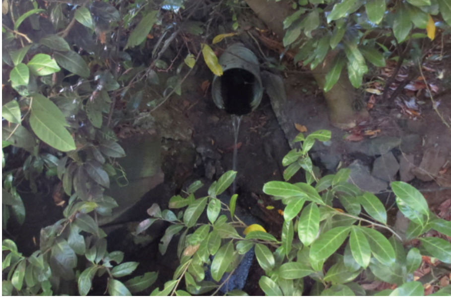
Figure 5. A stormwater outfall into the Kingfisher Natural Area, formerly Thornton Creek Park #2. Photo by author.
