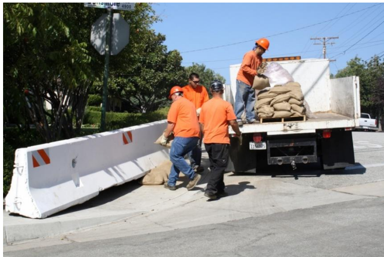
Figure 2. K-Rail being installed in La Crescenta, CA. Photo courtesy of Crescenta Valley Weekly.
