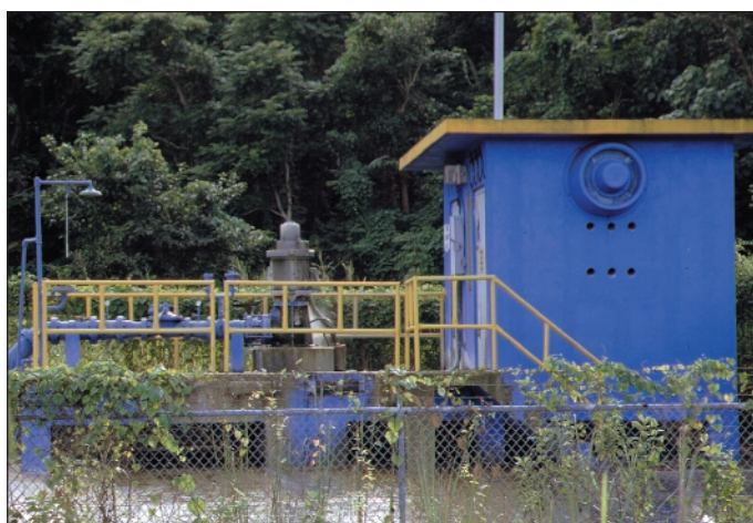
Photo 51. The Puerto Rico Water Company's ground water pumps in Dorado, Puerto Rico. Photo by L. Miranda Castro.
