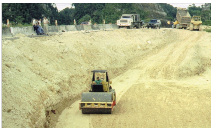
Photo 61. Maintenance activities in Highway PR 10. The road had already been officially opened when this picture was taken. Continuous landslides make it unlikely that this level of maintenance will ever abate in this road segment. Photo by L. Miranda Castro.
