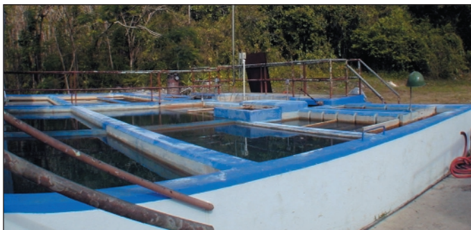
Photo 52. Cordillera potable water treatment plant in Ciales, Puerto Rico. Photo by L. Miranda Castro.
