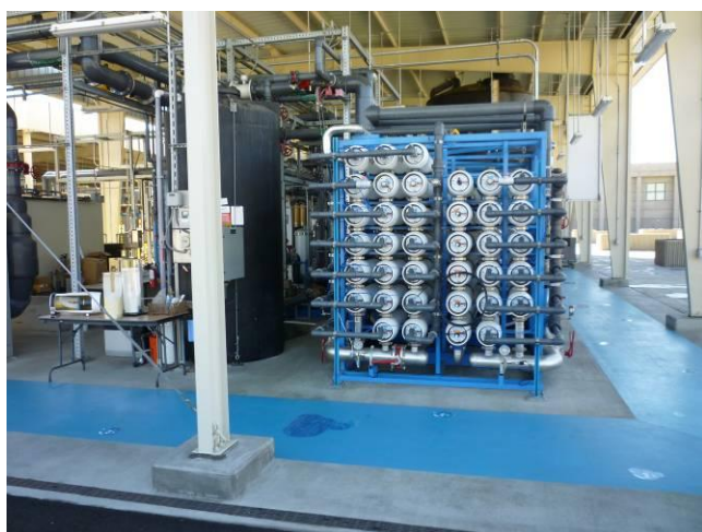
Microfiltration and reverse osmosis treatment area.
