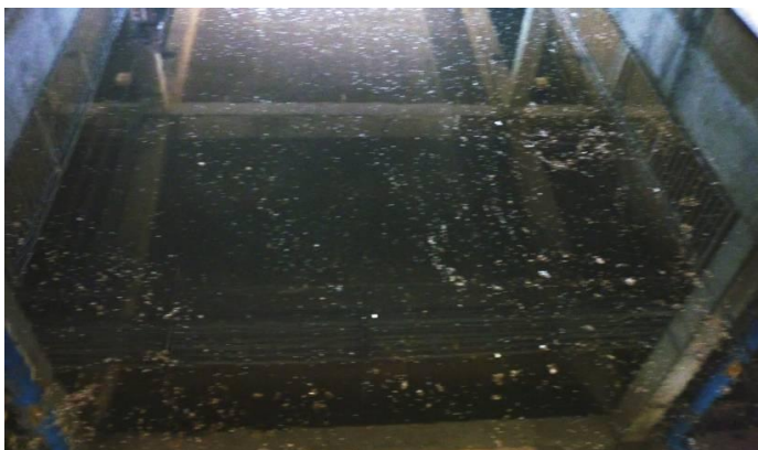
Carbon filtration stage
