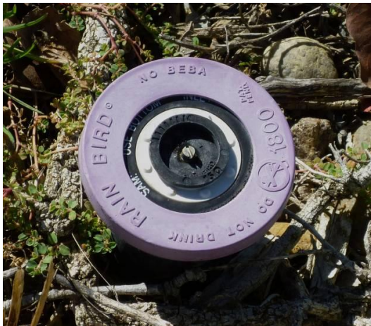
Purple coloration required for marking sprinkler heads using non-potable water.
