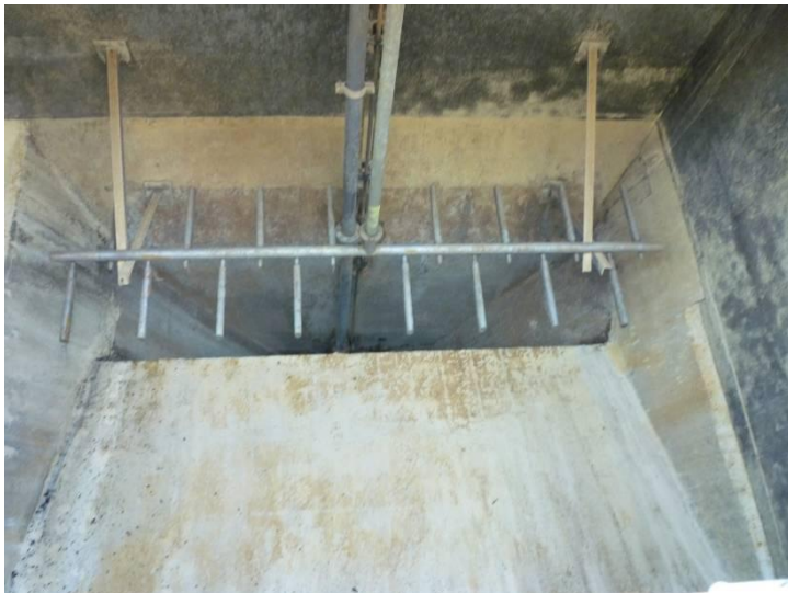
A second filtration step removes grit. Above is an image of the empty grit-removal machinery. The pictured bar rotates, which agitates the water and forces the grit to settle as the lighter water remains above.
