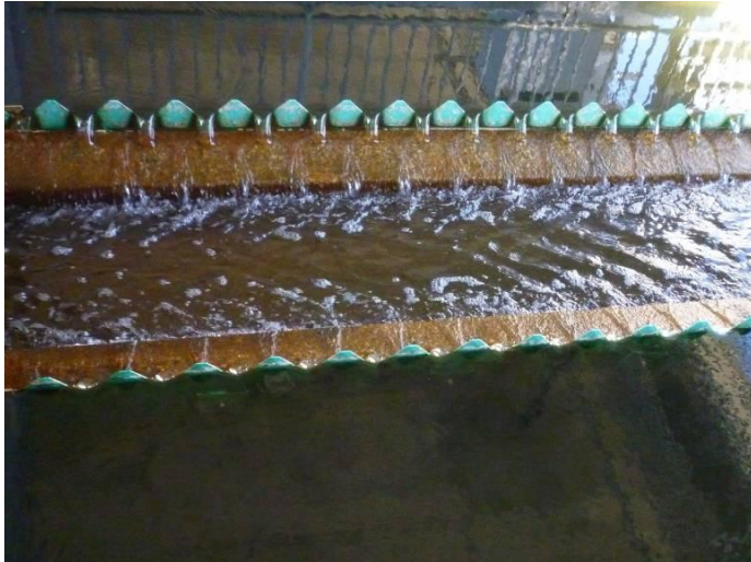
Nitrate and nitrite removal stage. Anaerobic bacteria feed on these chemicals.
