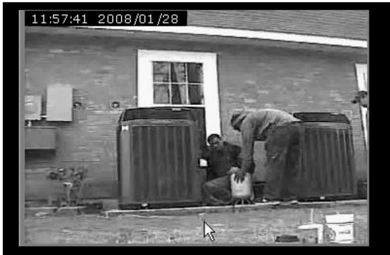
Figure 5. The SightPros communication tool captured three technicians installing new condensers at a customer site. Luis talked with Kwame. Oscar watched on the right. The video also showed power bank panels 2, 6, and 7 on the left.
