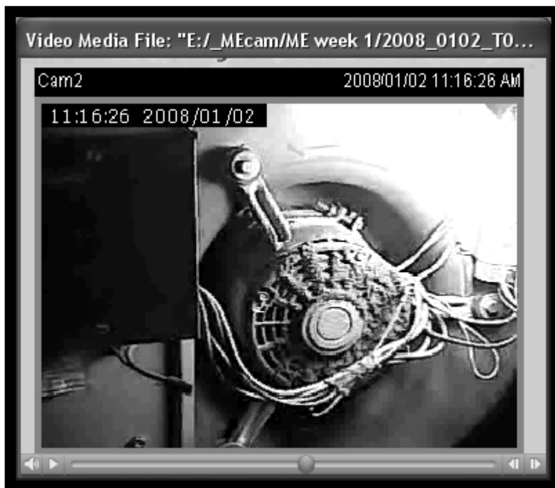
Figure 8. John viewed this dirty, noisy blower motor in a remote, almost dark attic.
