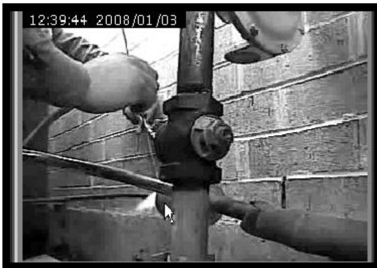
Figure 7. Luis carefully followed safety precautions as he soldered a connection with an open flame torch. He worked next to a gas line, a gas meter, and a drier exhaust vent in a very tight space between a bush, a condenser, and a brick house.
