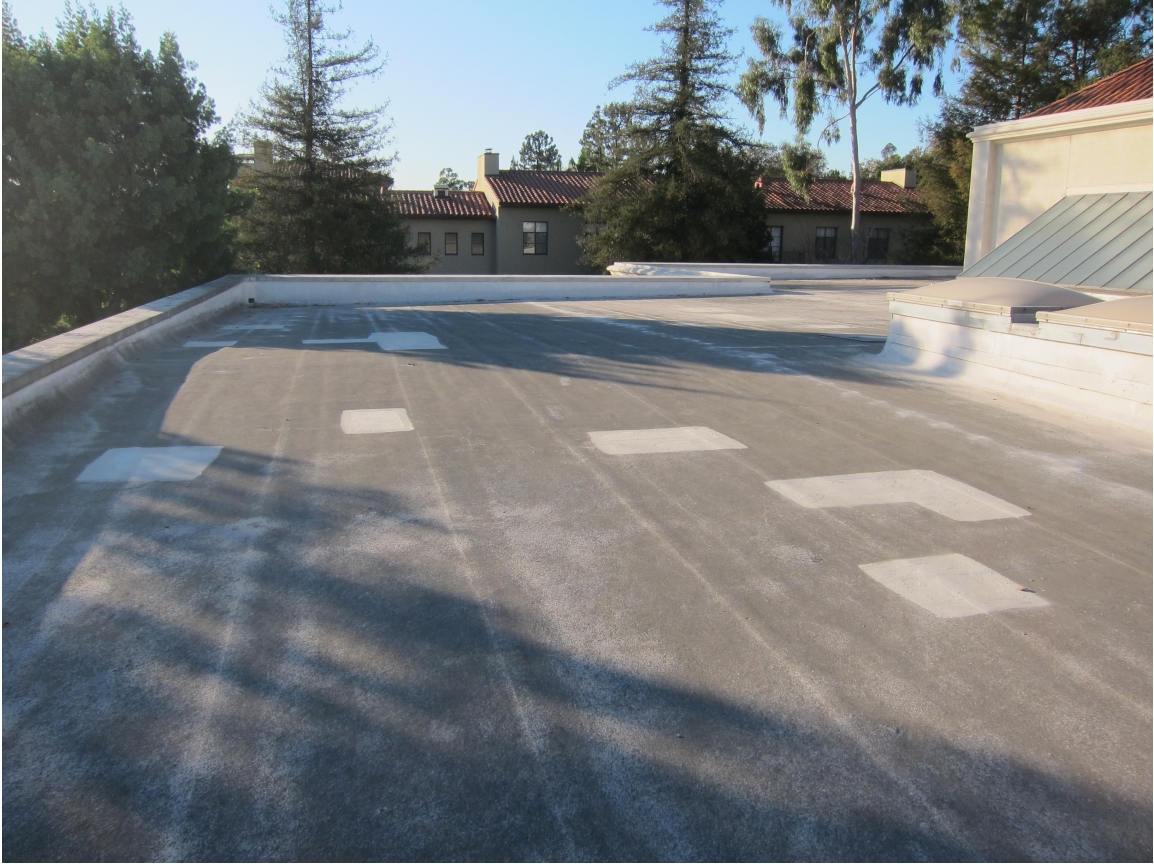
(Fig 19) Frank dining hall has a single-ply reflective coating that as can be seen has aged significantly. This coating is laid down as a continuous sheet, and so even a small tear can cause leaks. This is the reason for the several light colored patches. (12/6/11)
