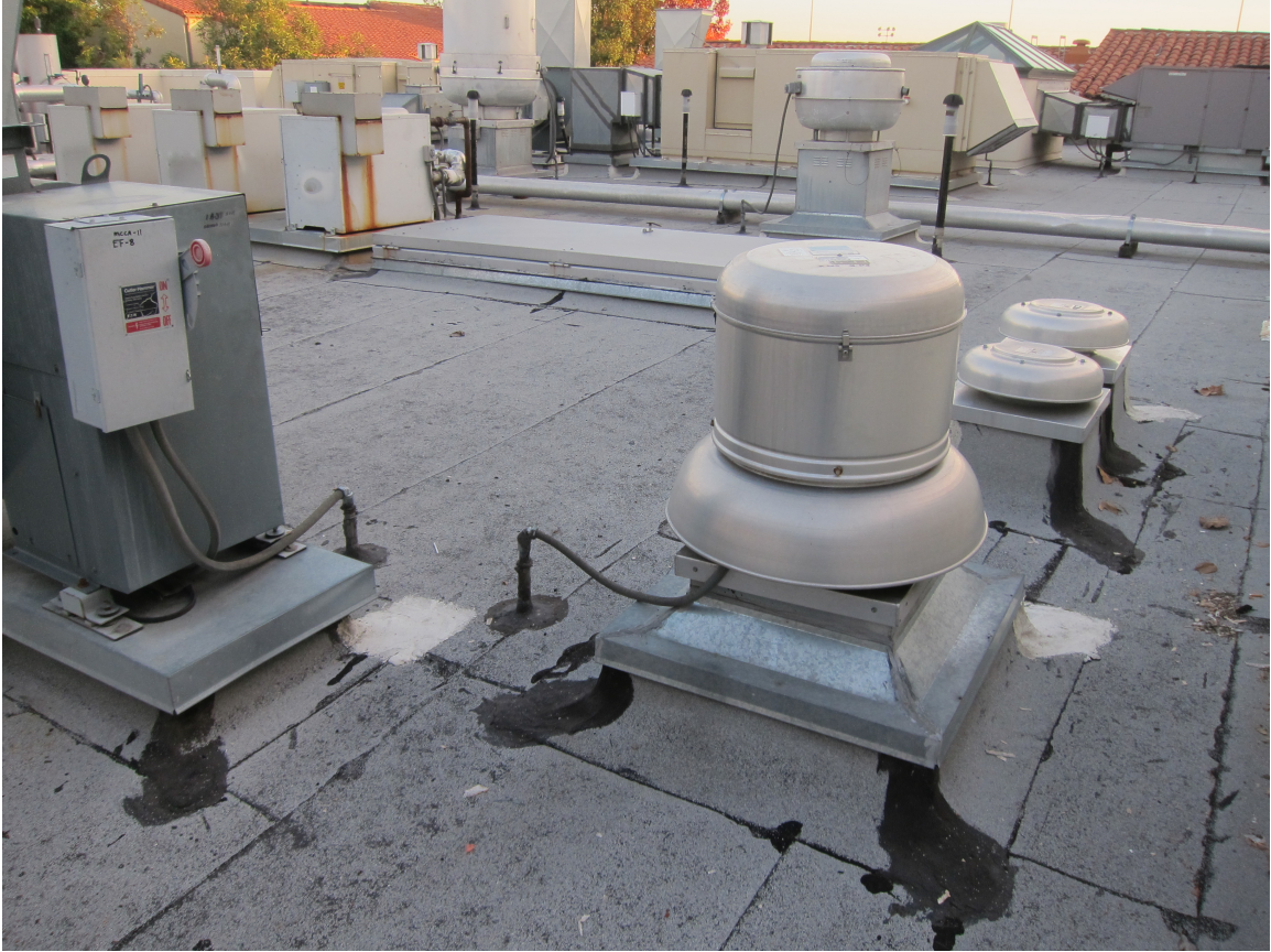
(Fig 17) This is the flat roof above the kitchen of Frary dining hall and it features a built up coating of layered asphalt and polymer sheets. The coating on this roof is not a reflective coating, but due to the evident age of this coating it could be due for resurfacing. At this point a reflective coating should be considered. (11/30/11)
