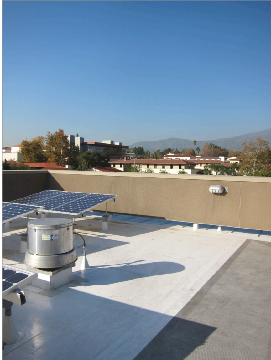
(Fig 21) This is the new single ply reflective coating on top of Sontag Hall. It is similar to the coating on Frank, though it is much newer. (11/30/11)
