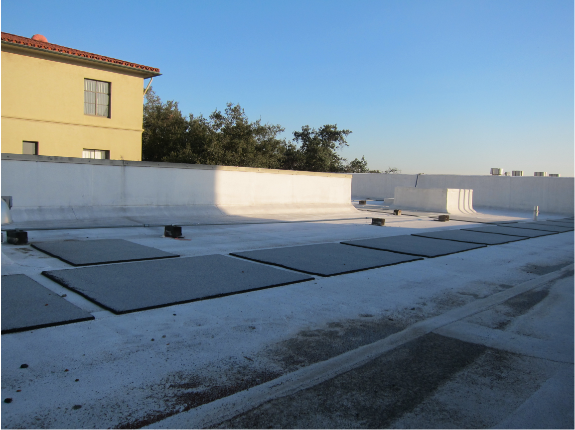
(Fig 16) This is the roof on top of Gibson dorm. It features a liquid applied reflective coating, though it has lost some of its brightness due to age and dirt accumulation. This effect can be seen in the difference in color between the walls and the deck. (11/30/11)
