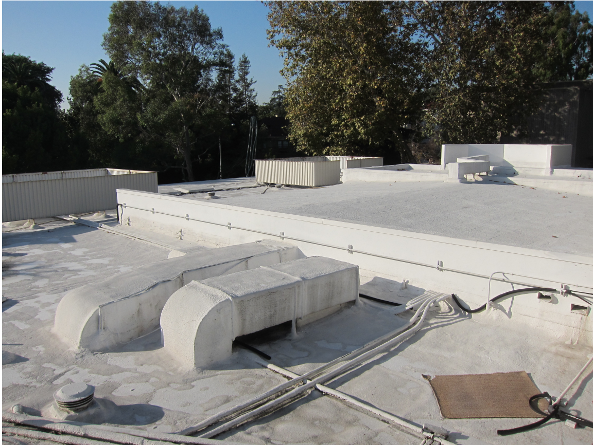
(Fig 13) The flat built up roof on top of the art museum is covered with a high albedo coating. This coating is comprised of reflective granules and as can be seen in this picture is sprayed over roof surfaces and can also cover ventilation ducts. This is also a foam roof, which according to the manufacturer provides additional energy benefits over a standard concrete roof. (11/30/11)
