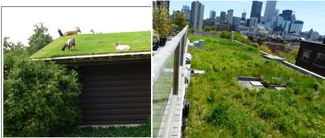
(Fig 9) Green roofs can reduce energy use, reduce air temperature, and reduce runoff. They can also be designed as usable roof top garden space and bring a lot of value through human enjoyment. A green roof is also a great place to keep your goats. 23
