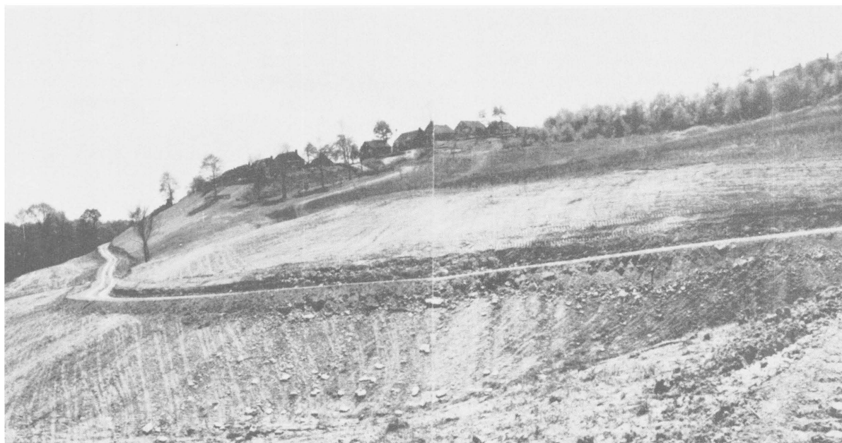
FIGURE 35.—Typical Inspection-Maintenance Road Constructed Over Surface-Sealed Area. (Road also provides surface drainage.)
