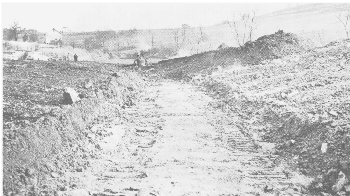
FIGURE 54.—Trench Made To Isolate a Soil Fire, Which Will Be Back-Filled With Incombustible Material.
