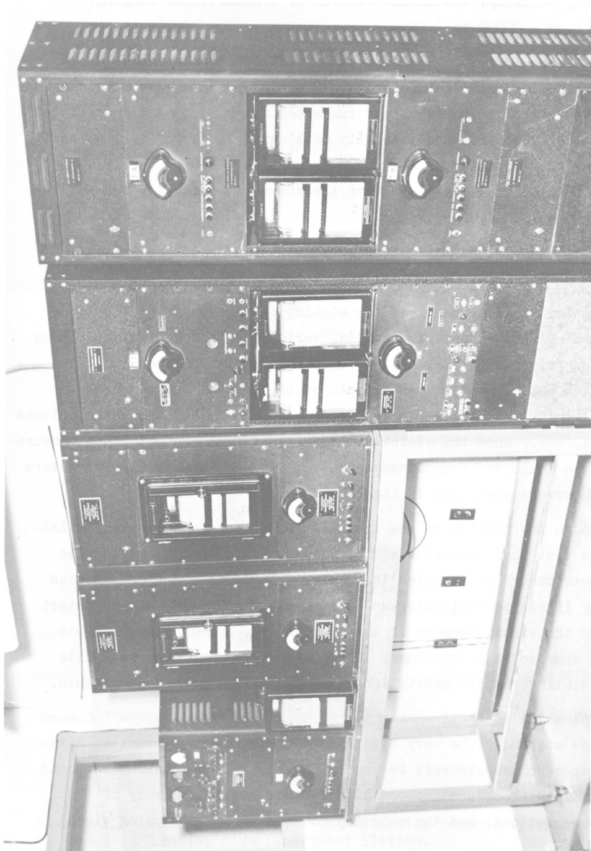
Figure 3.6 Central transmissometer recording position at the Landing Aids Experiment Station. The signal to the instrument in the extreme left was transmitted by UHF radio.
