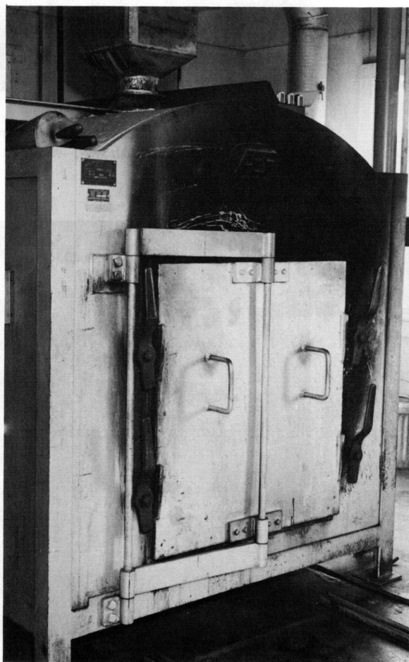
Figure 5. Gas fired furnace for normal uranium scrap burning (see Table 3). Note tracks on floor on which a hood with exhaust ventilation can be rolled up to the front of the furnace, so that the trays in the furnace can be pulled out into the hood.
