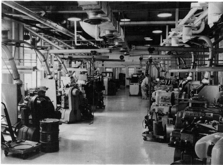
Figure 3. Normal uranium machine shop (see Table 2). This shows the old shop after local ventilation was installed; note the flexible ducts extending down to the machines.
