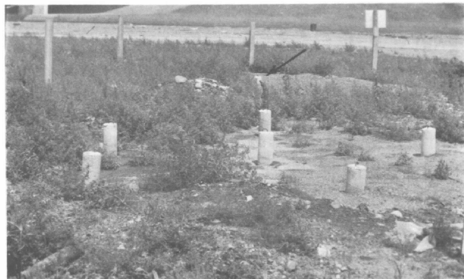
FIGURE 2. Site C—View (after backfilling) showing concrete caps covering the reinforcing rods. Location of the horizontal pile is indicated by arrow in the background.
