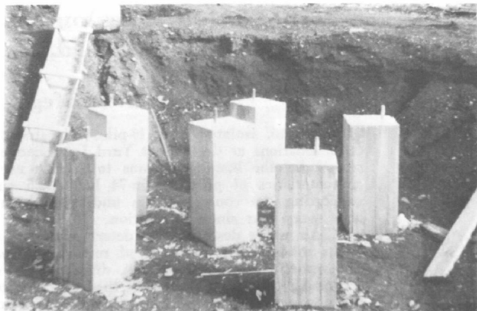
FIGURE 1. Site C—View (before backfilling) showing the 6 driven piles encased by concrete at the upper ends. Reinforcing rods shown protruding above the concrete are for the electrical connection.
