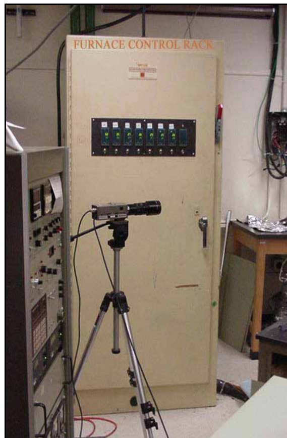
Figure 24. Furnace control unit housing rack.
