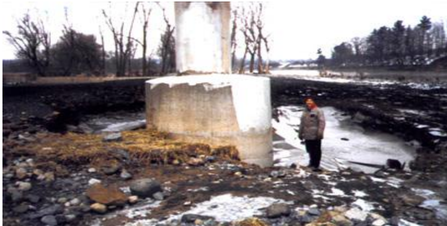
Figure 2-4: Scour at I-90 West Pier.
