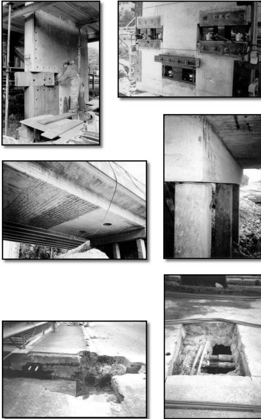
Figure 5-4: Photographs illustrating the applied damage scenarios. From left to right and from top to bottom: (1) cutting of a pier to install the settlement system, (2) settlement system, (3) spalling of concrete, (4) failure of a concrete hinge, (5) failure of anchor heads, (6) failure of tendon wires.
