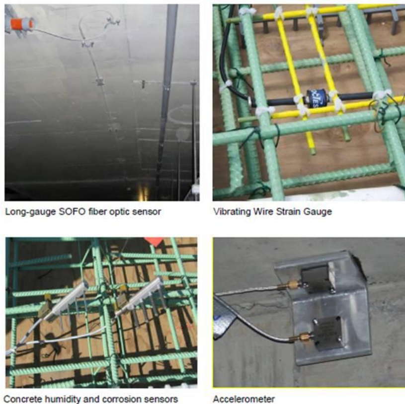
Figure 2-7: Sensors installed in the I-35W Bridge.
