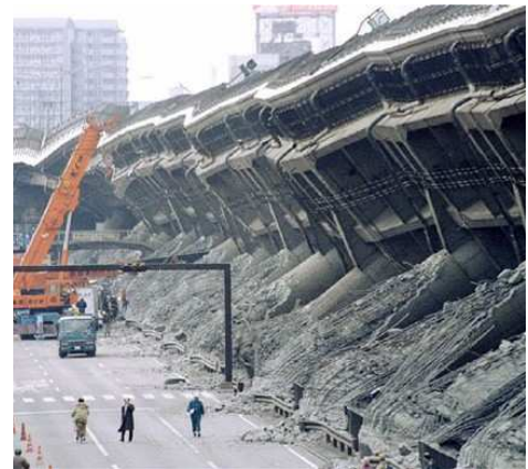
An highways collapsed in Nishinomiya, between Osaka and Kobe (Warner, 2011)
