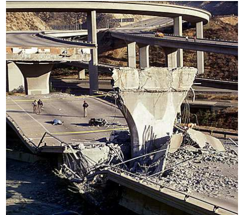
The California State Route (SR 14) fallen over the Golden State Freeway (I 5) (Los Angeles Times, 2012)
