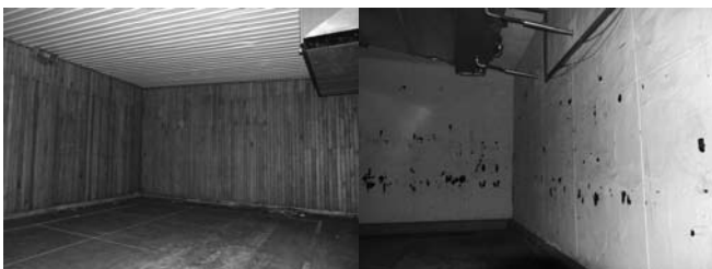
Fig. 2. Detail of two of the small cold chambers before demolition (the first with ICB protected by wood; the second with painted ICB).
