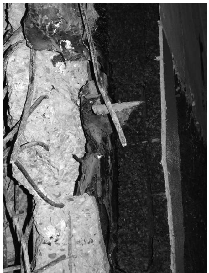
Fig. 5. Detail of the wall of one of the big cold chambers (reinforced concrete, asphalt sheet, two ICB layers (15+10 cm) and covering).
