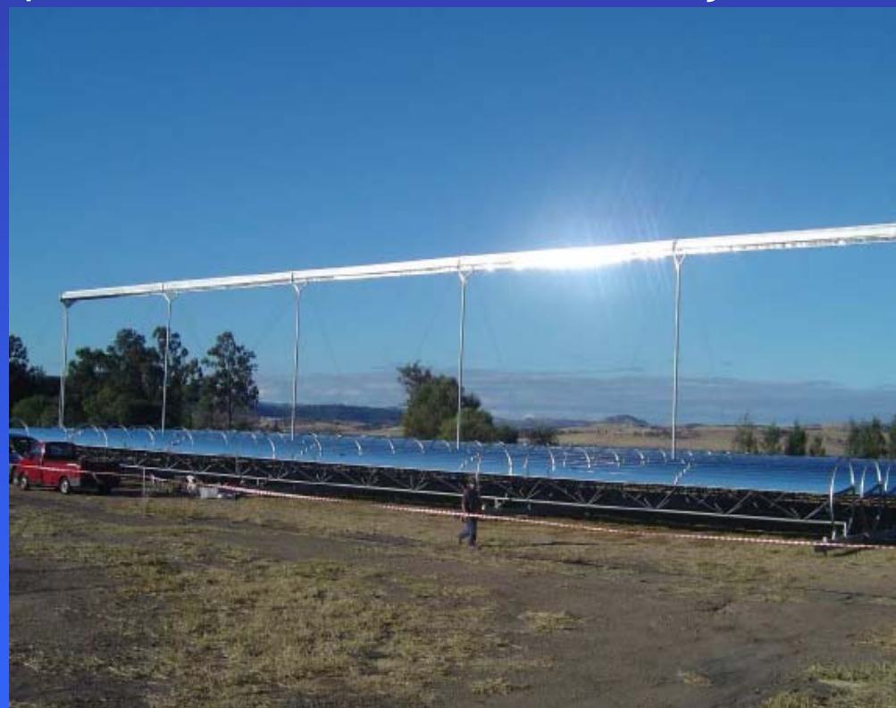
centrais do tipo Compact Linear Fresnel Reflector 6 MWp
