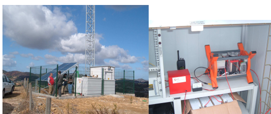
Fig.1 AEA demonstration project site. Fuel cell installation is also shown.
